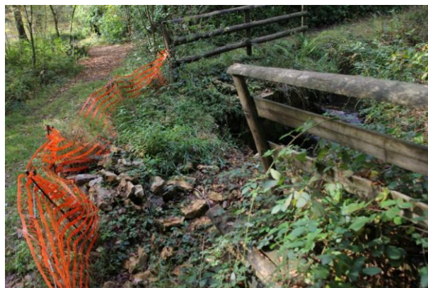
The broken culvert in the Victorian leat which will be repaired.
